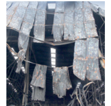
Roof sheeting hanging from severely deformed steelwork.
