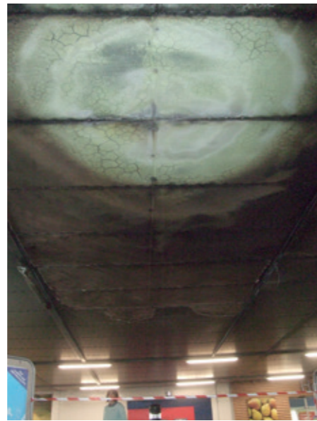
Evidence of direct flame impingement on soffit lining directly above the car.
