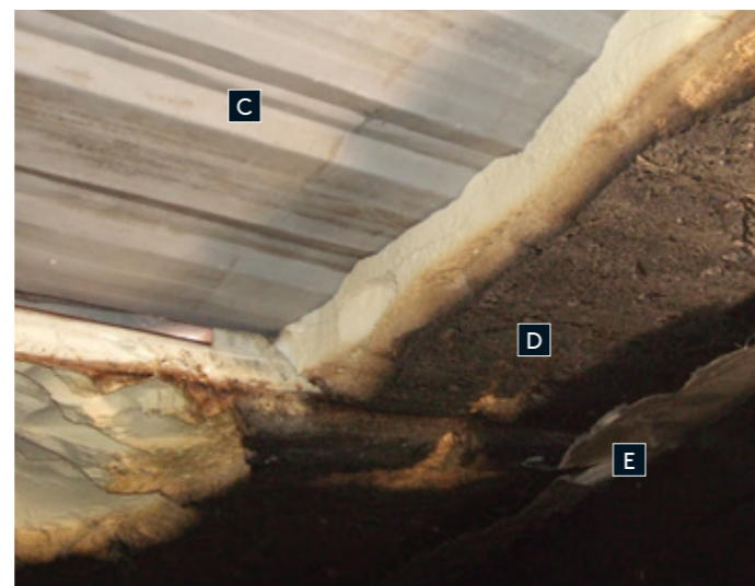
C: Temporary roof covering over hole in roof. D: PIR core showing delaminated lower surface and extent of through-thickness charring. E: Cut edge of lower steel skin of sandwich panel.
