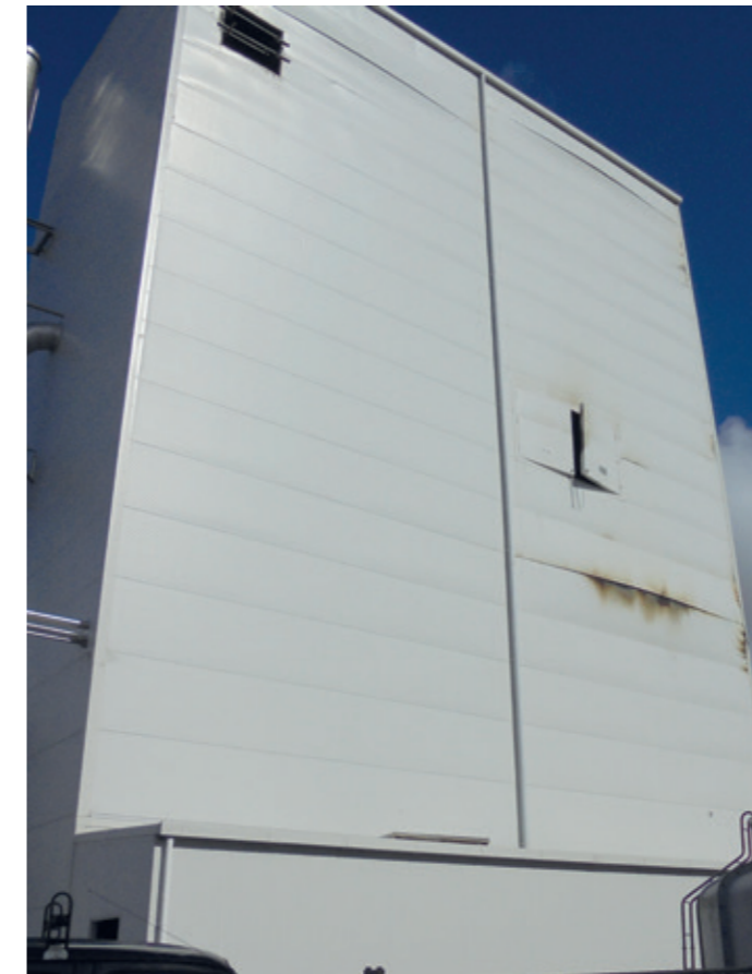
Milk powder drying tower showing external fire damage to panels explosion doors opened manually after fire).
