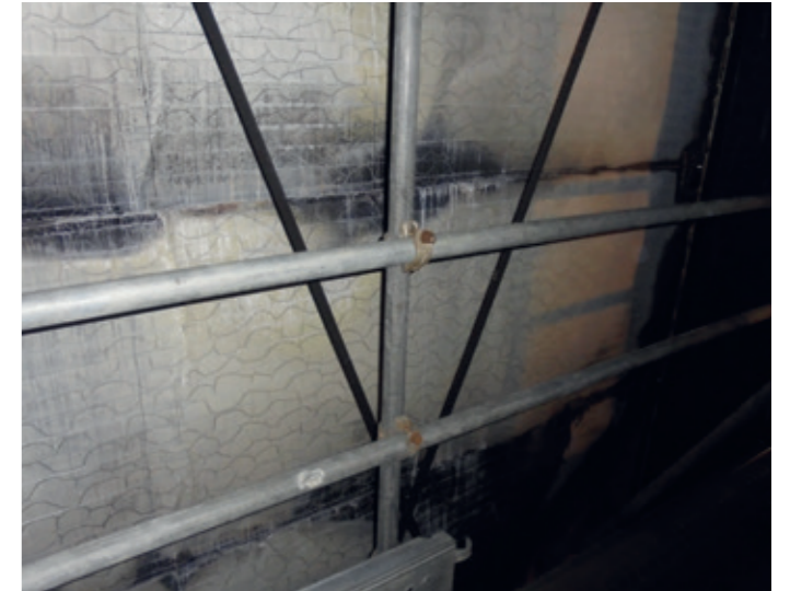
Panels exposed to fire internally.
