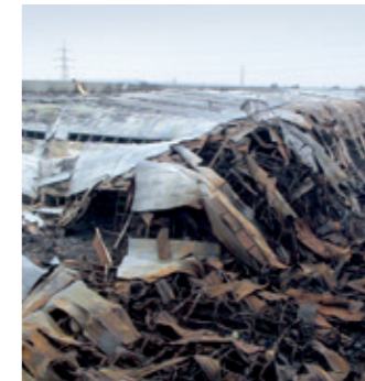
Collapsed south end of building.
