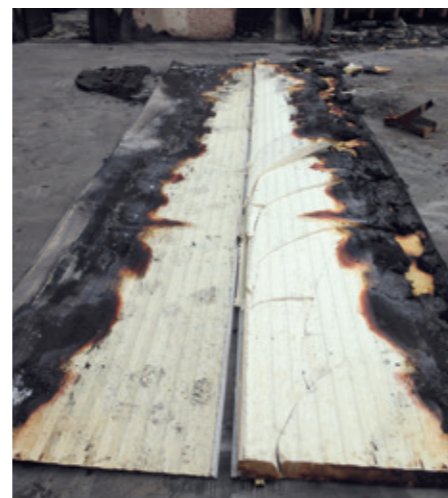
Panel at junction with steel stripped off demonstrating charring of PIR core but no evidence of fire spread.
