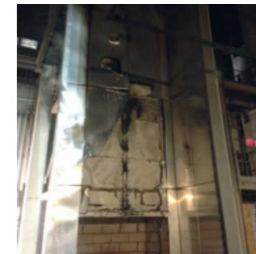
End of test showing aluminium cassette melted away to expose underlying Kingspan BENCHMARK Karrier panel in place
