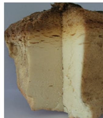
Insurer Approved PIR core sample showing extent of through-thickness charring at Suffolk Food Hall.
